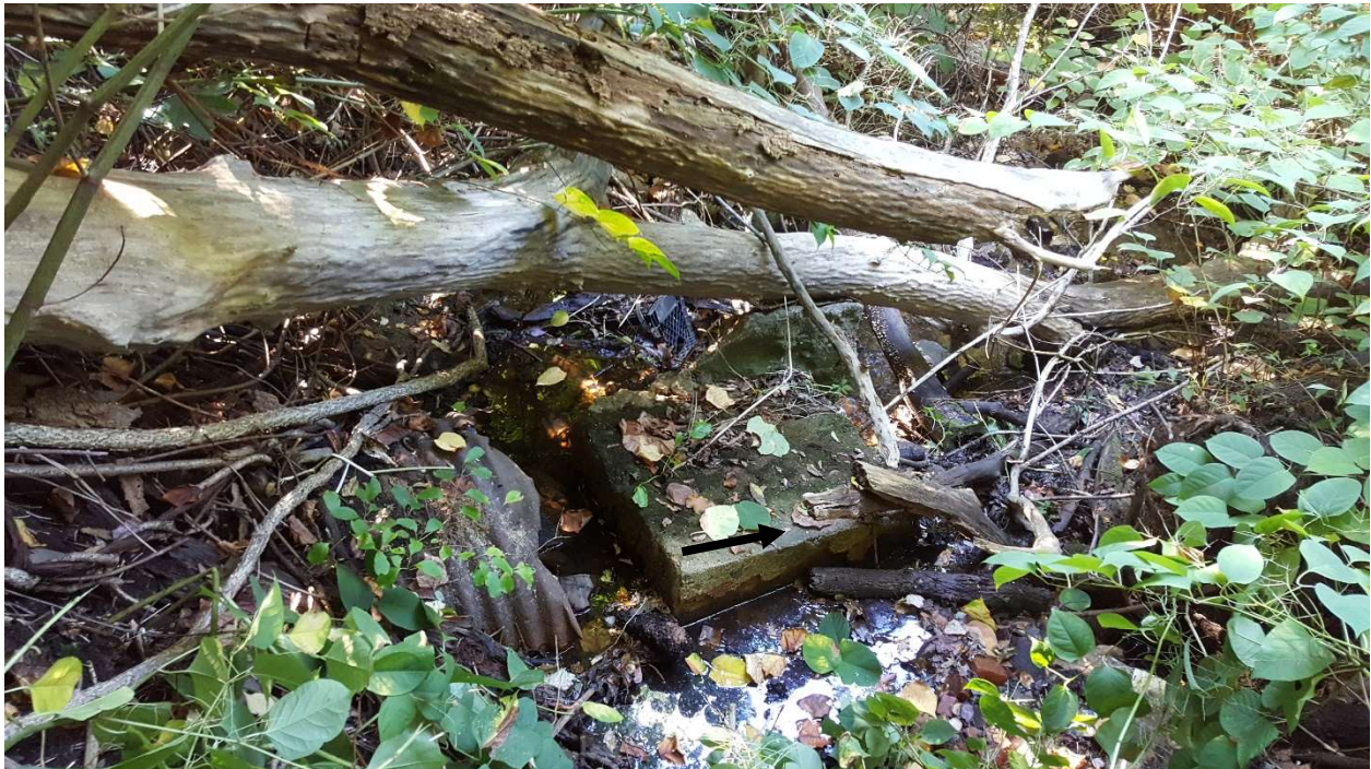
Figure 7. Corrugated metal pipe, which is the outlet of Titus Pond and the beginning of Buttery Brook. Outlet is perched and severely deteriorated. Arrow indicates flow direction. Looking east near flag E501.
