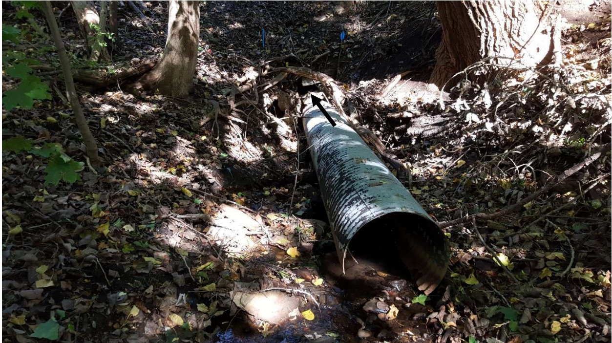
Figure 15. Outlet for Buttery Brook south of Mountain Avenue. Arrow indicates where majority of flow emerges from crossing, as pipe segments have separated. Looking northeast (upstream).
