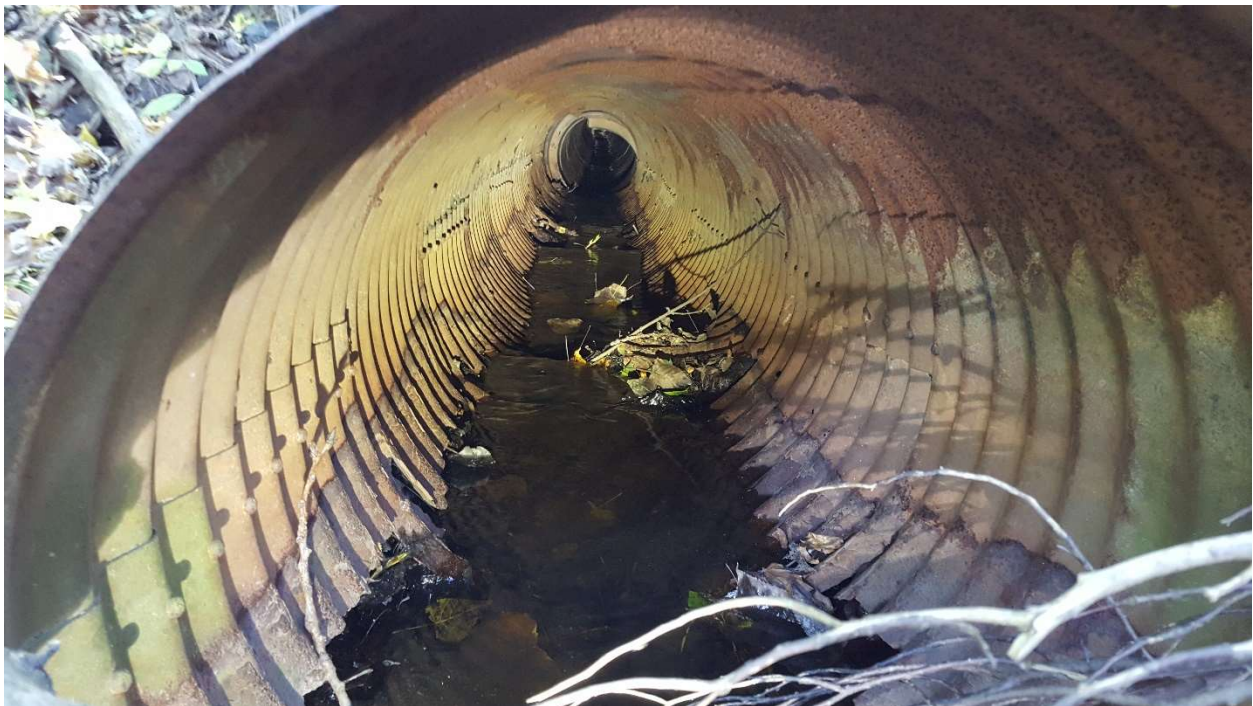
Figure 14. Deteriorated culvert conveying Buttery Brook under Mountain Avenue. Looking south-southwest from the inlet north of the road.
