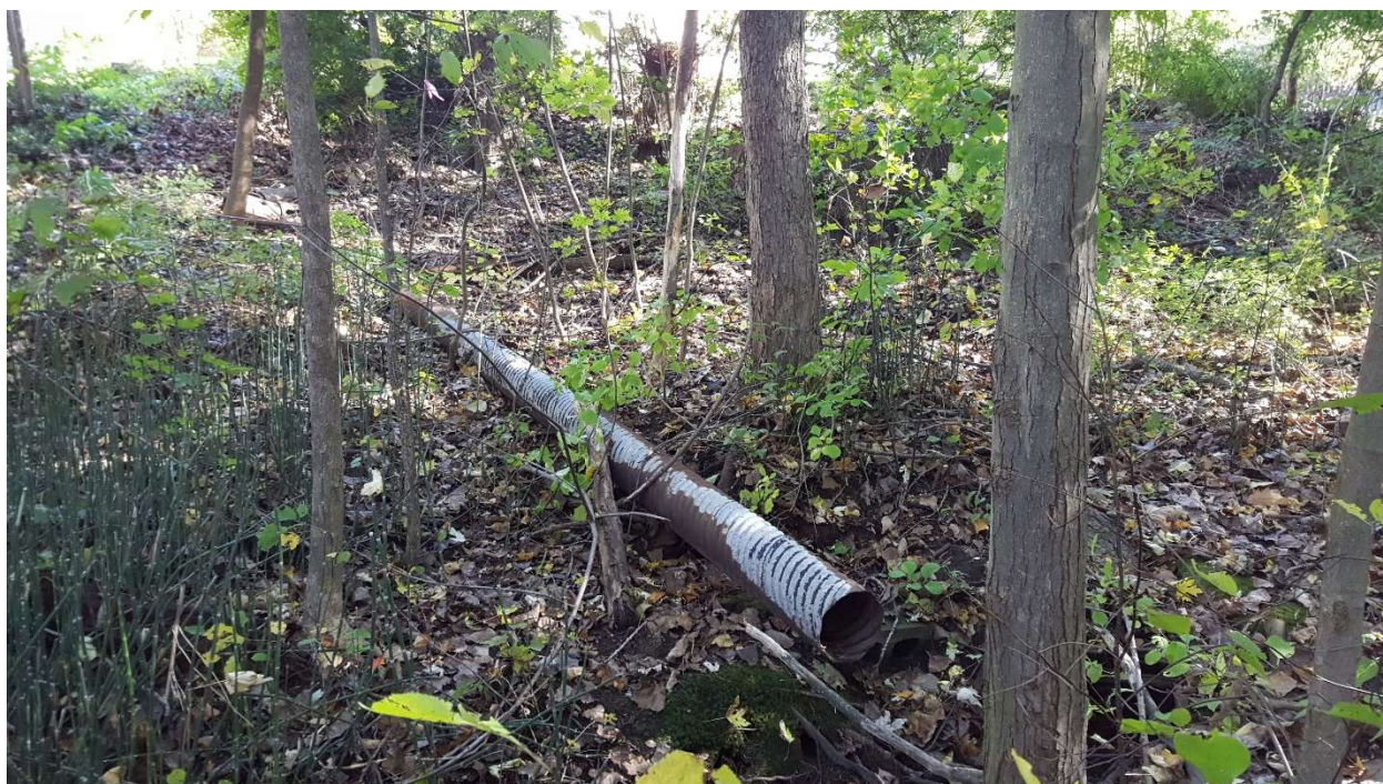
Figure 4. 8-inch corrugated metal pipe, presumably a stormwater outfall, within the BVW along the northern bank of Titus Pond (flag series B200-B215). Looking north.
