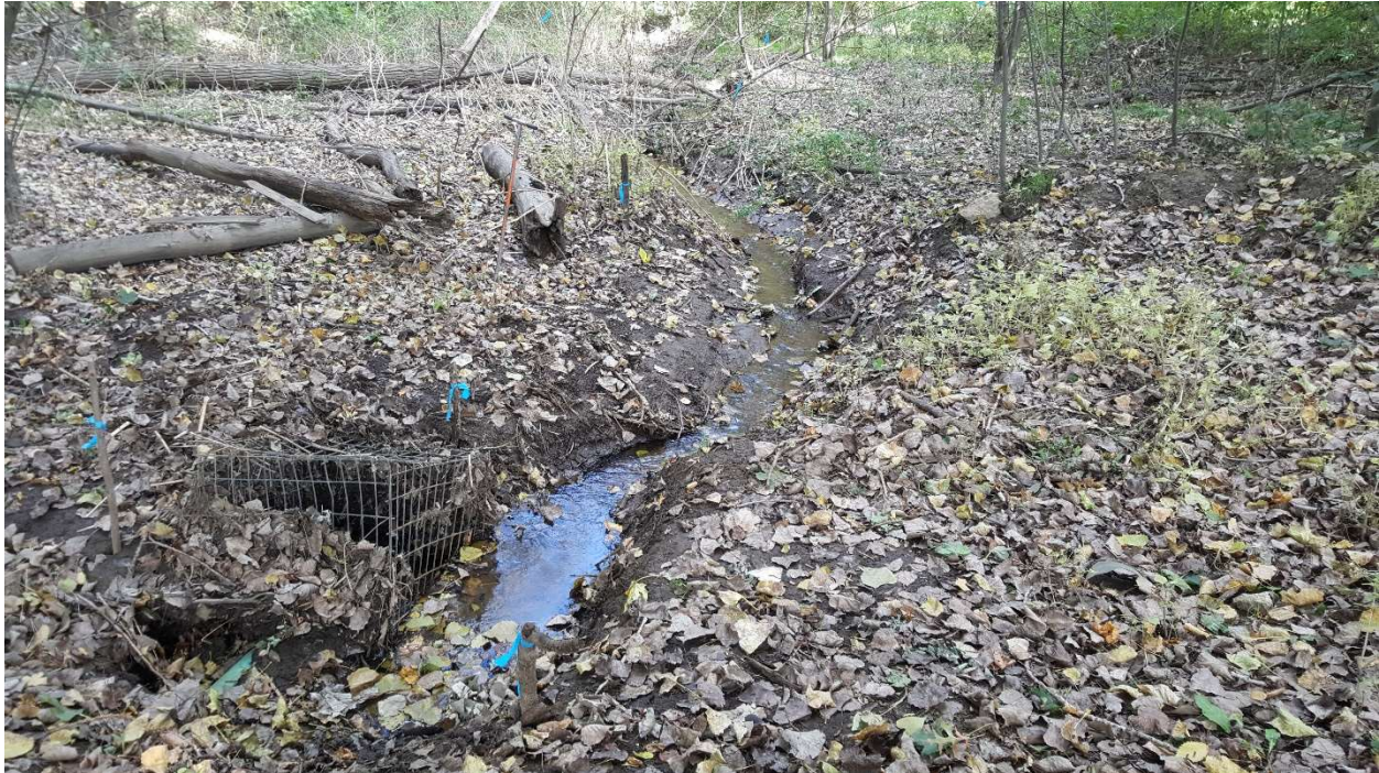
Figure 21. Buttery Brook and inlet to the buried reach under Joffre Avenue and surrounding area. BVW (flag series K200-K213) encircles the inlet and is visible at right and left. Looking northeast (upstream) near flag F656.
